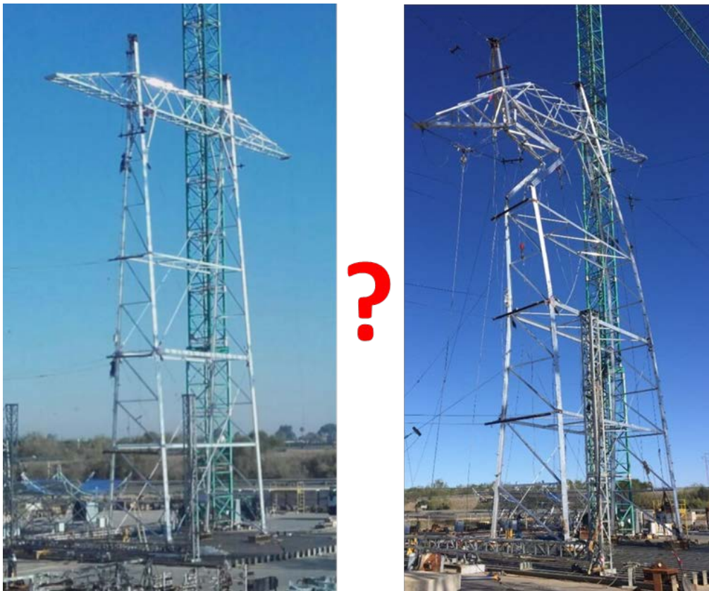
Fig. 1: Pictures of the tower prior to testing as well as after collapse in the final test.
